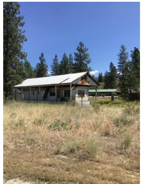
Trailer home with flammable siding .
